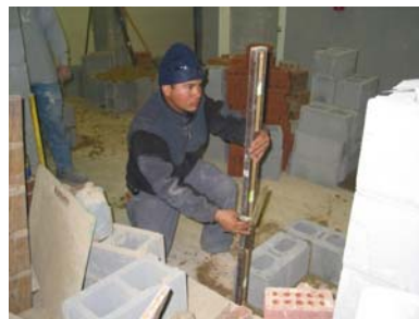
Alfredo Cervantes with Bibler Masonry works hard to pass Stage Five hands– on project.
