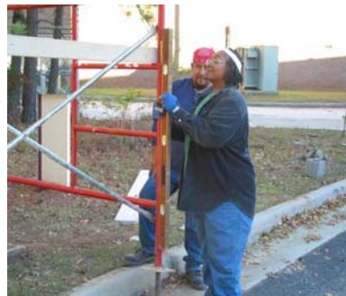
Scaffold building is an important skill for Stage One students to master before they can move on to Stage Two. Charlie Reeves & Hector Rangel demonstrate proper technique.
